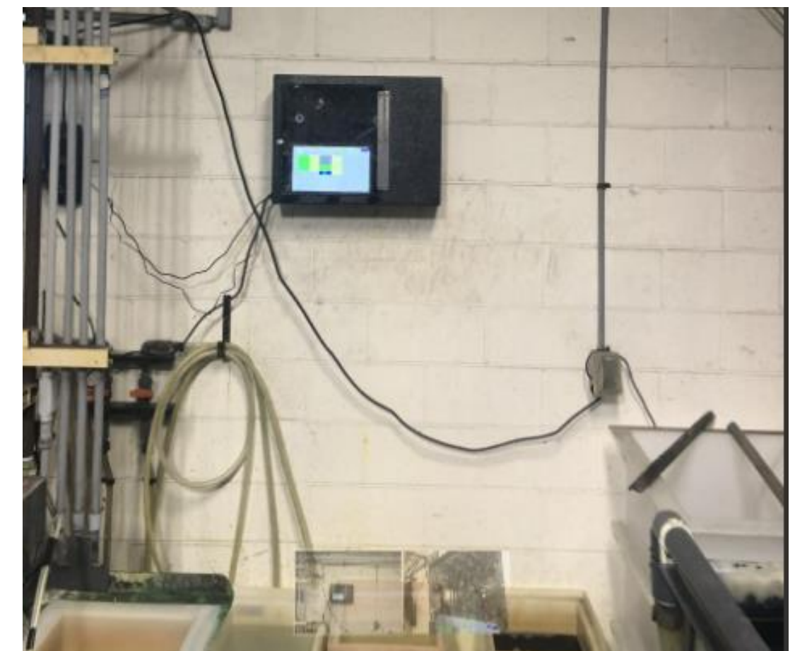
Installed Dust Shield Enclosure with a Wall Mount [2]
